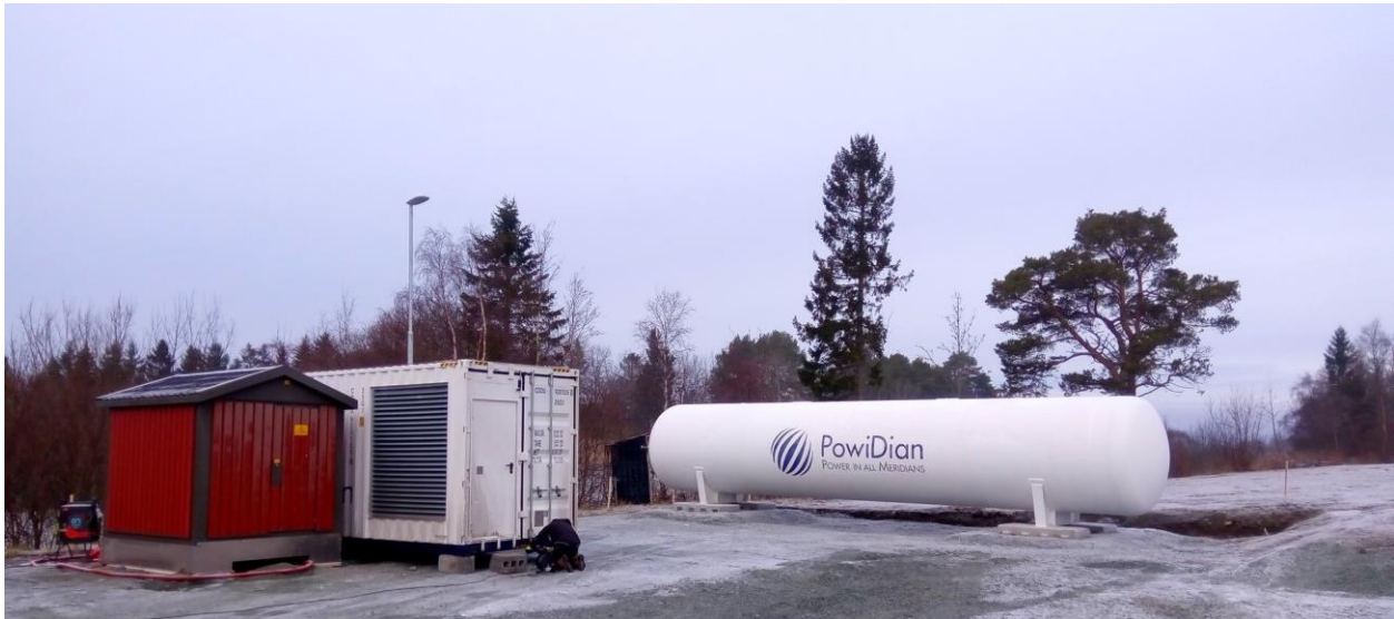
The fuel cell container and the hydrogen tank are ready to be started in Rye, Norway.
